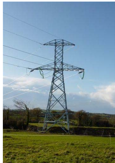
Plate 4.11 Typical Steel Angle Structure
